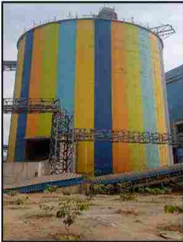
Clinker storage silo
